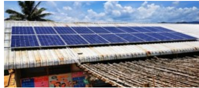
Solar Cell System 5.3kWp
